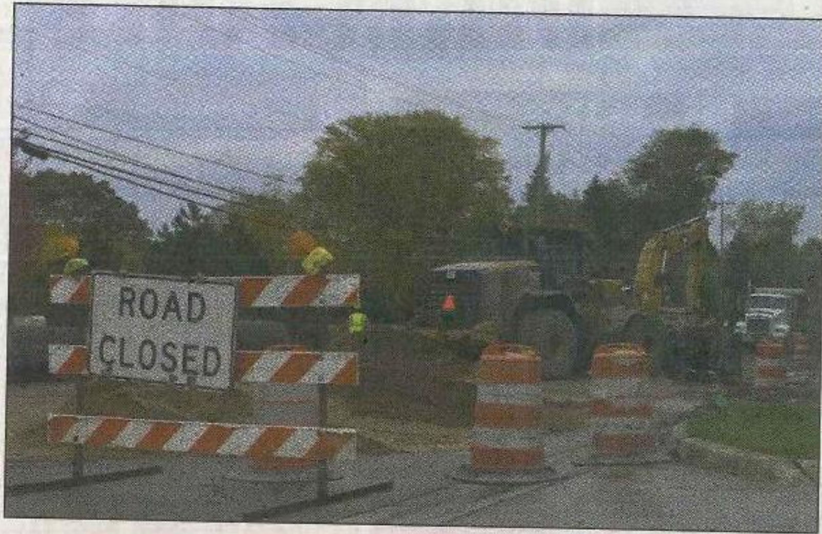
Officials from the Road Commission for Oakland County and the Macomb County Department of Roads recently announced plans for the reconstruction of Dequindre Road in Shelby Township, Sterling Heights, Troy and Rochester Hills. ADVISOR & SOURCE FILE PHOTO
